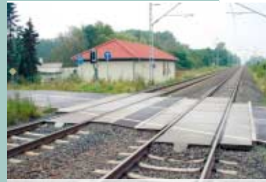
Rail crossing RAILBETON, Calbe
